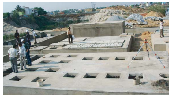
Completed DEWATS plant ready for inauguration
